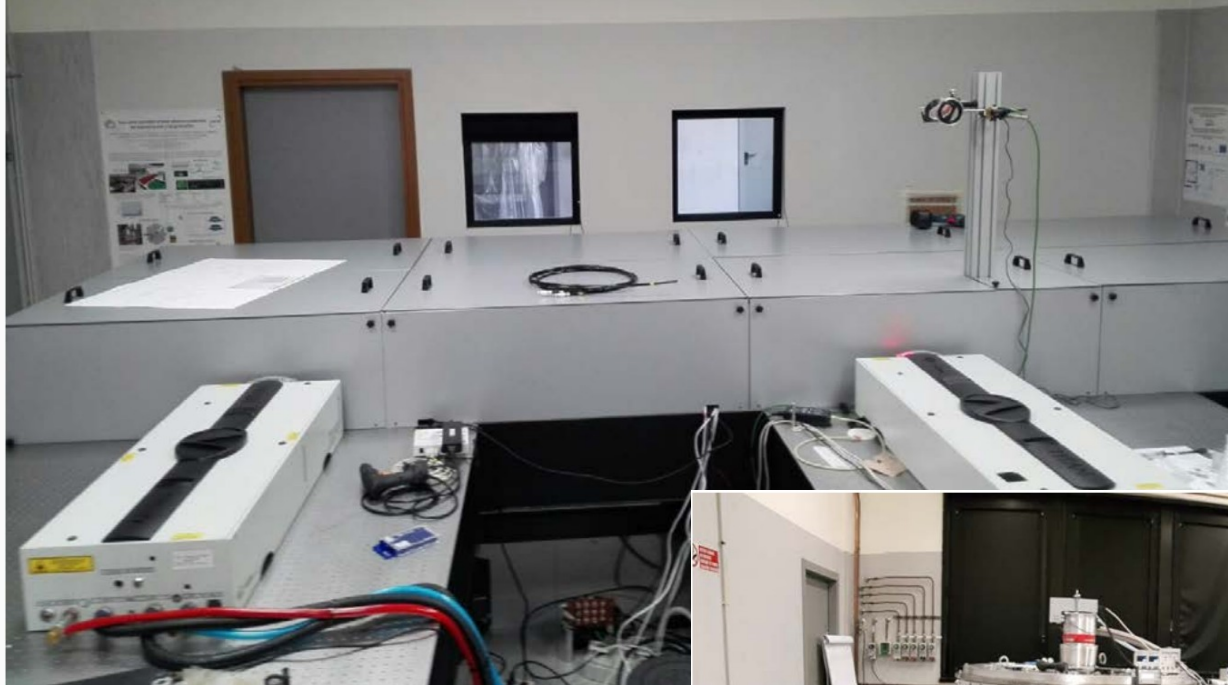
Final amplifier room
